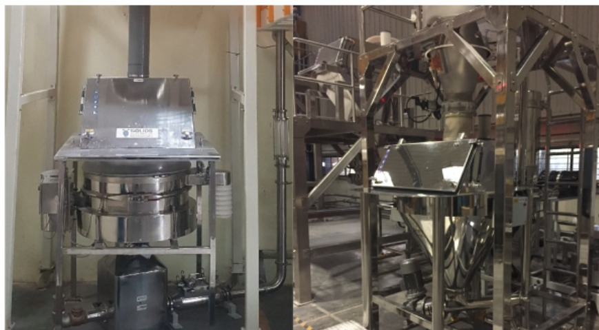
Bag Unloading Stations
